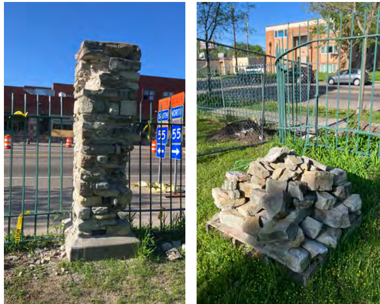
Work on the pillars of the Cemetery’s fence has begun. Built in 1928, the fence has been in need of substantial repairs for at least a decade. Some of the soft limestone blocks and the mortar that held them together for almost 100 years need to be replaced. The restoration will take several months and is expected to be completed by fall.
